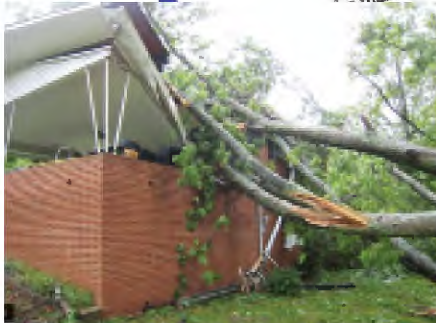
Trees brought down by high winds collapsed a car port on National Director Kay Pearson's home in Tennessee.
